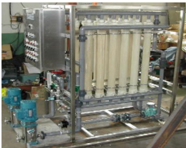
The Micro Membrane Filtration System of the ISWM facility
